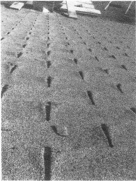
Photo 3 – pronounced separation between shingles
